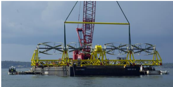
ORPC's TideGen unit being readied for installation at Cobscook Bay, Maine. From www.orpc.co .
