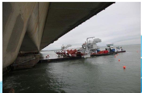
Installation of five turbines in progress at the Eastern Scheldt Barrier. From www.pro-tide.eu .
